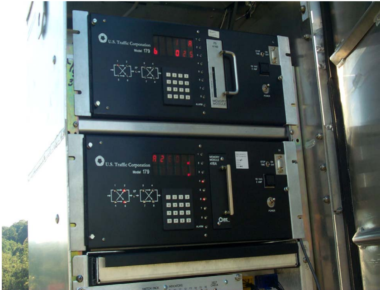
U.S. Traffic Corp. Traffic Signal Controller
